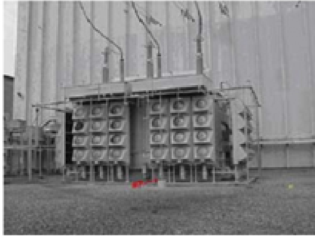
Main Power Transformer Image with Oil
