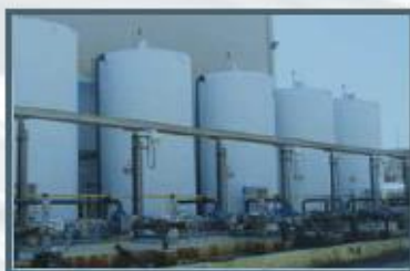
Bulk storage tanks
