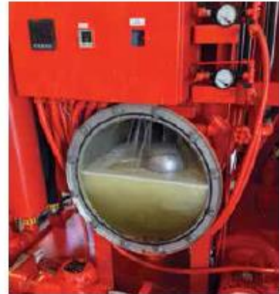
Vacuum dehydrator used to remove water contamination.
