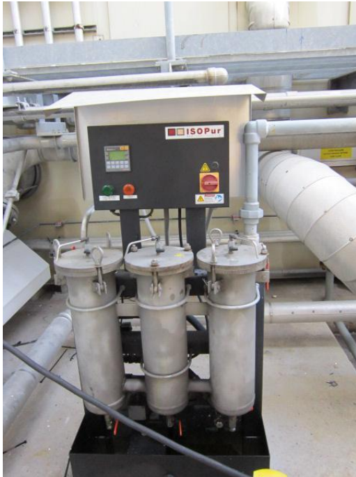
Figure 1. MR installation on a GE 7FA Turbine Oil Sump
