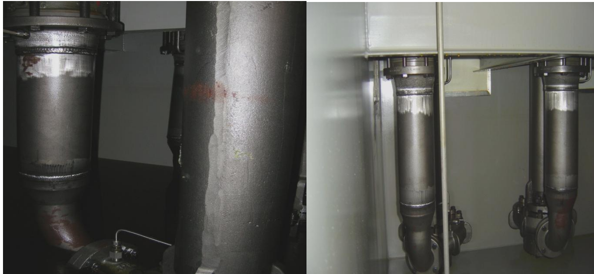
Figure 8. Oil Tank after Nine Years of Operation
