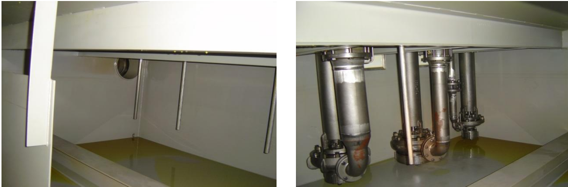
Figure 3. Oil tank internal inspection at 20 weeks after installation
