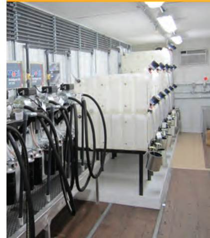
The TEP lube room
